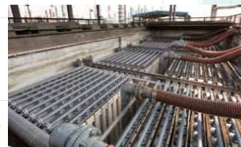
Water treatment system introduced at a large Taiwanese oil refinery
